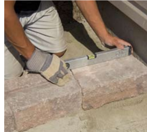
THE FIRST ROW OF BLOCK IS BURIED. THIS ROW NEEDS TO BE PERFECTLY LEVELED.
